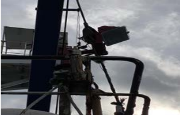
Starboard side emergency light near life raft unlit. [inoperative]
