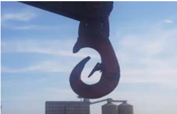
Davit hooks found to be corroded and stuck in an open position. [Not properly maintained]
