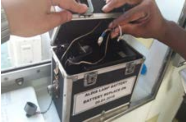
Daylight signaling lamp cannot be tested with emergency source of power supply
