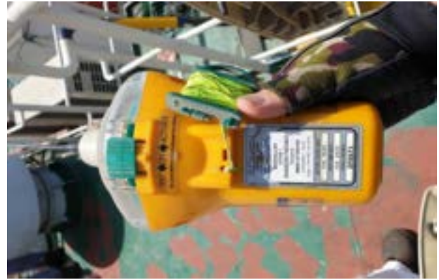
EPIRB battery is expired. [Not as required]
