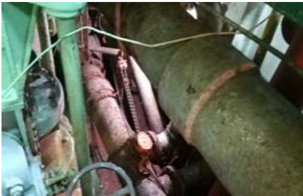
Main ballast valve from sea chest hanged with chain block
