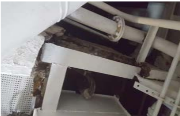
Asbestos in one part of the engine room ceiling (beside the emergency exit) is not properly isolated.
