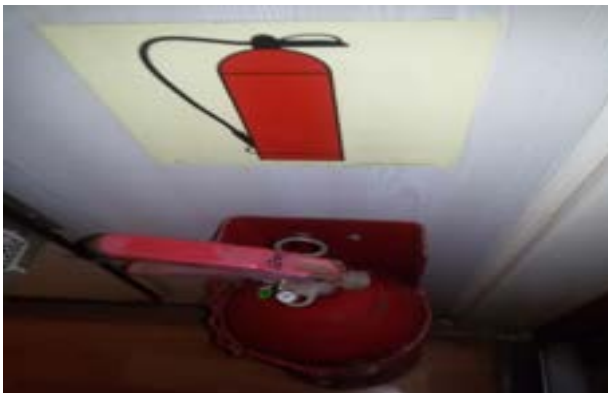
Nozzle of portable fire extinguisher next to gyro room removed
