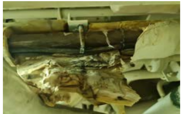
One steam pipe from engine room found with temporary repair
