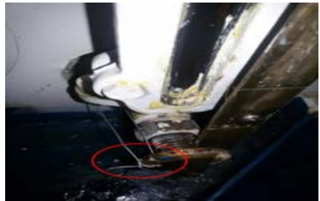
Sight glass v/v of m/e fuel tank fasten tight and open.
