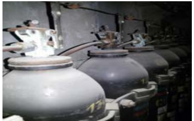
Co2 room lighting in poor condition and 2 bottle heads sulphated. [Incomplete]
