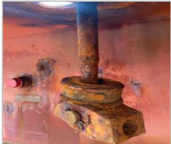
Hatch cover cleats corroded [corroded]
