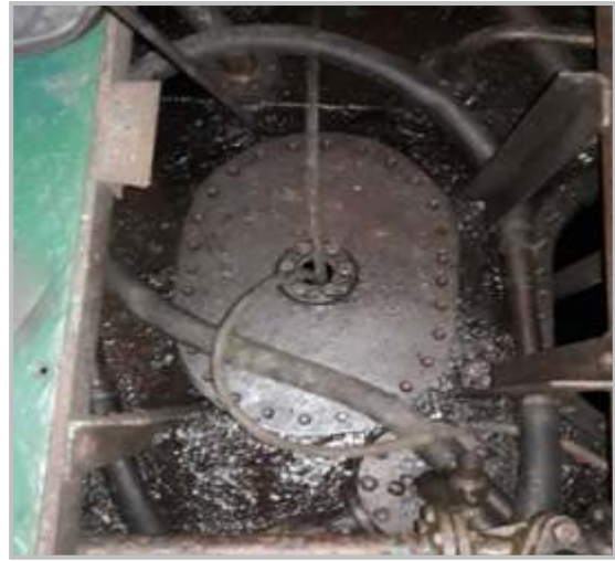
Sounding pipe of fuel leakage tank in e/r removed & fuel lines connected to tank irregularly. [improperly used]
