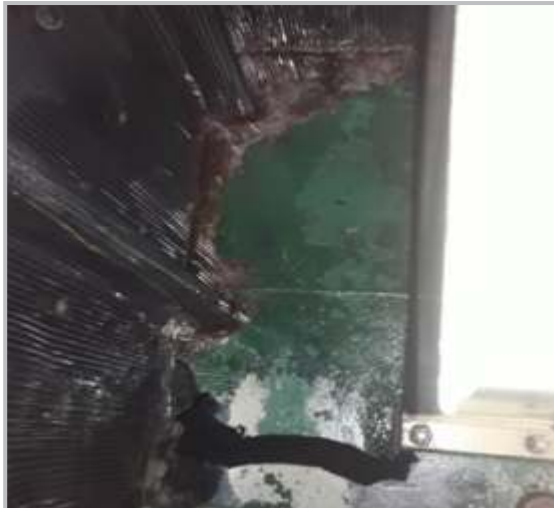
Slippery floor due to hydraulic oil leakage in steering gear room. [slippery]
