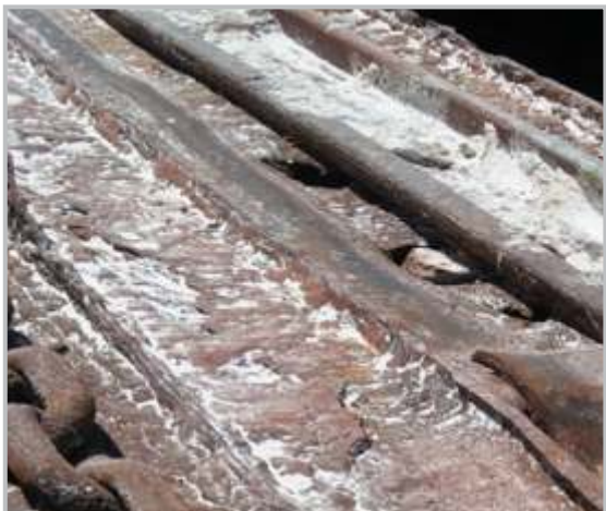
Cargo hold hatch covers compression bar rusted & some parts went holes. [corroded]
