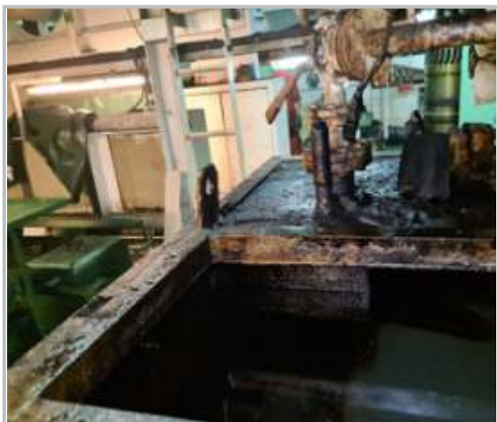
Oil and Oily mixture found in Cascade tank
