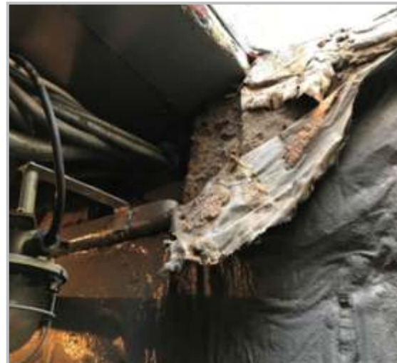
E/r emergency exit compartment bulkhead asbestos isolation was damaged. [damaged]
