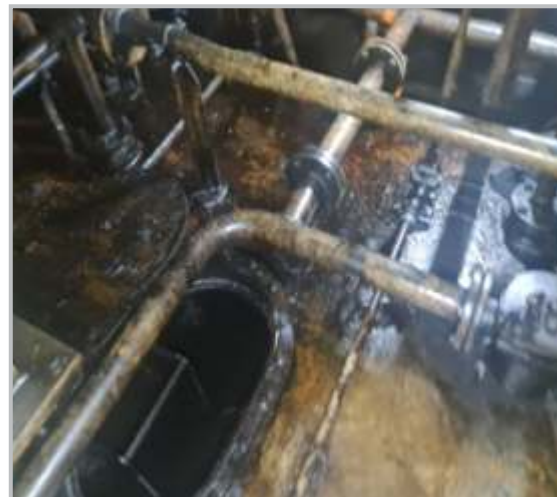
Oil and oily mixture found on tank top area and Aux Engine area [Lack of familiarity]
