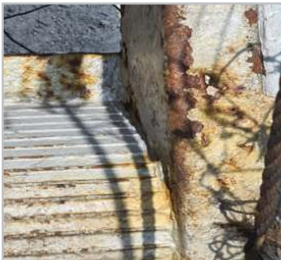
Found hole at accommodation ladder frame [not properly maintained]
