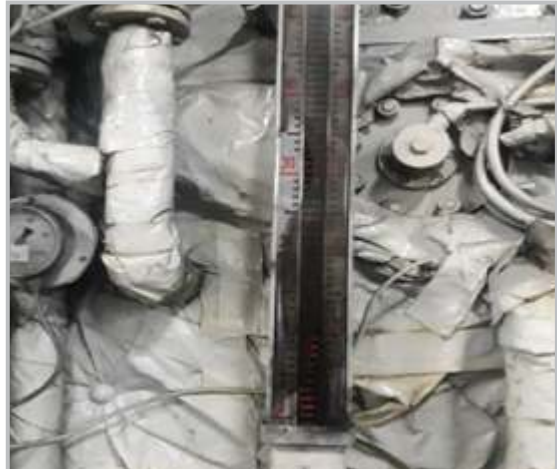
Sight glass of main fuel tank in e/r broken. [not as required]
