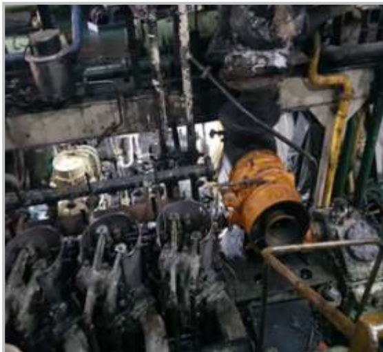
The Main Engine is out of order [missing]
